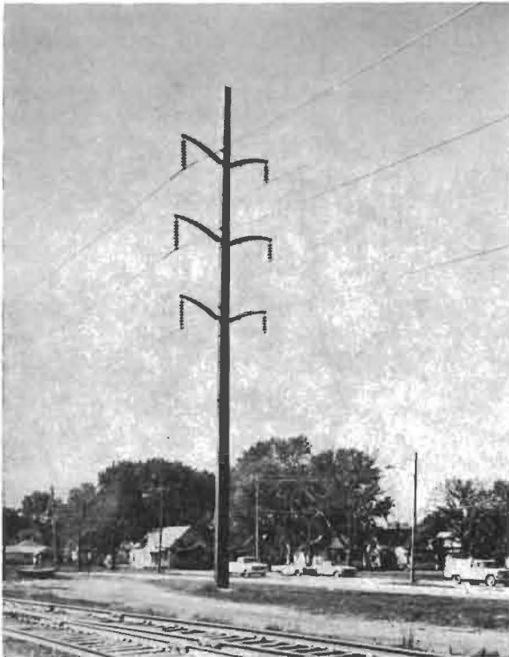
Figure 2.—110' Laminated Pole With Laminated Up-swept Side Arms 161 KV and 69 KV Circuits—Treated With Penta With "Light Colored" Heavy Oil.
